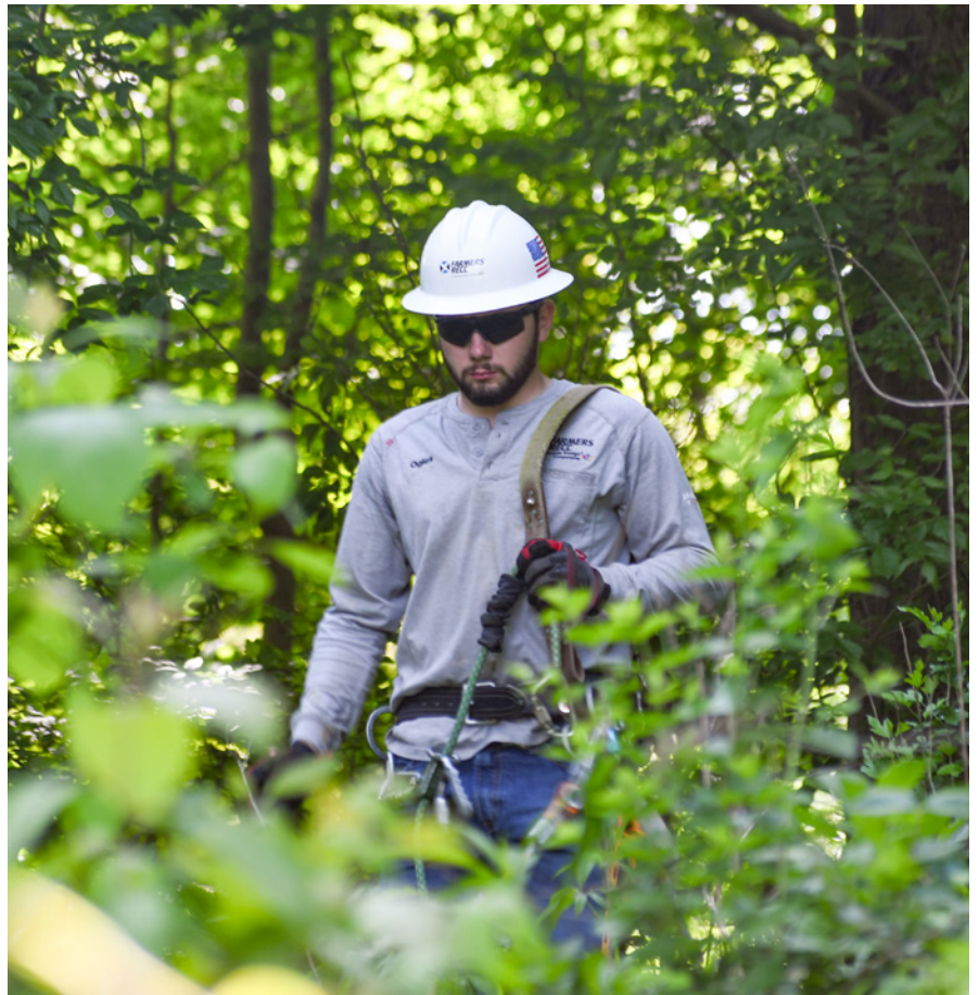
Apprentice lineman Taylor Ogles works on the Farmers RECC system to maintain and improve reliability. Photo: Abigail Nuetzman
